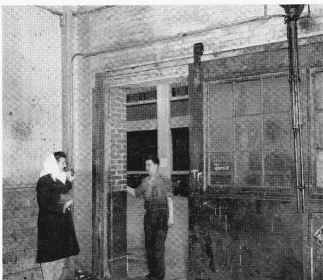
The many heavy doors around Scovill would be hard to handle if it wasn't for the air that's handy to do it for us. Charlie Novakowski presses the button so Ann Carpentier, Waterville messenger, can get through the big door at the North Mill. Either switch will operate the door.
